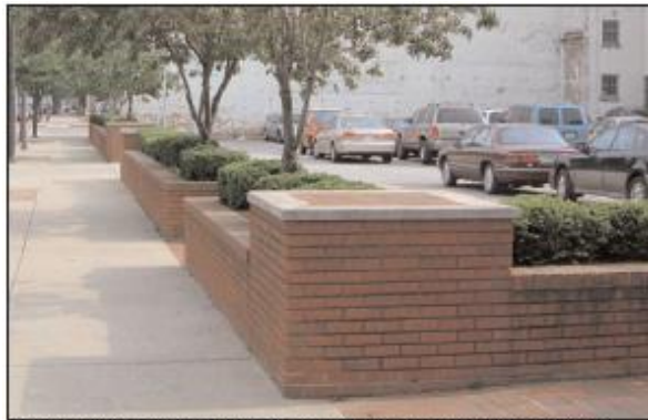
Existing seat wall and landscape planter in along Michigan Street in South Bend.
